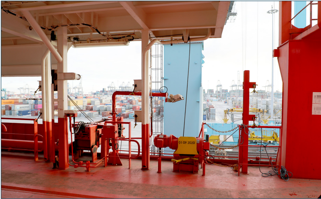
Figure 8: Gab in handrail by fall wire winch Source: DMAIB
